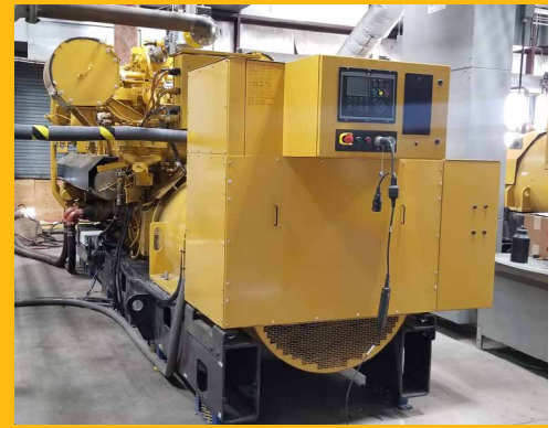
Heber Light & Power tests Cat® equipment pre-market.
